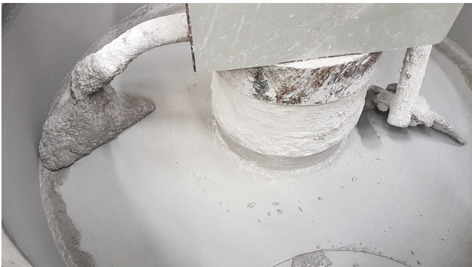
Not properly cleaned mixer!
